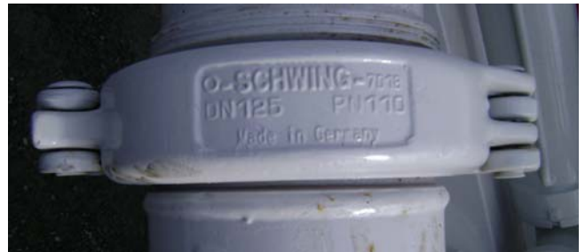
Photograph 4: An example of acceptable marking on pipe clamps.
