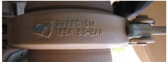
Photograph 3: An example of acceptable marking on pipe clamps.
