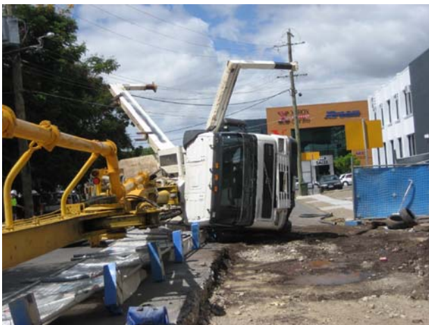
Photograph 1: overturned mobile concrete placement boom
